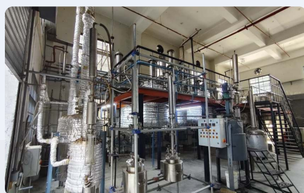
Fractional distillation columns
